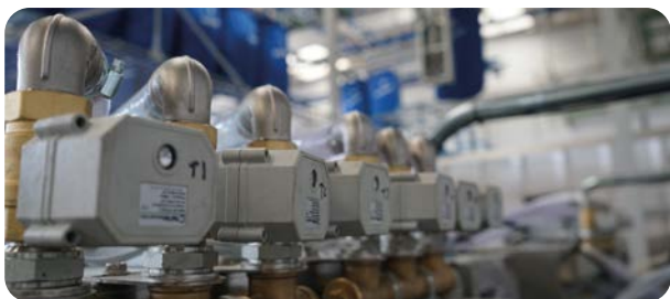
1" solenoid valves from tanks to washing machines and from pumps to tanks.
